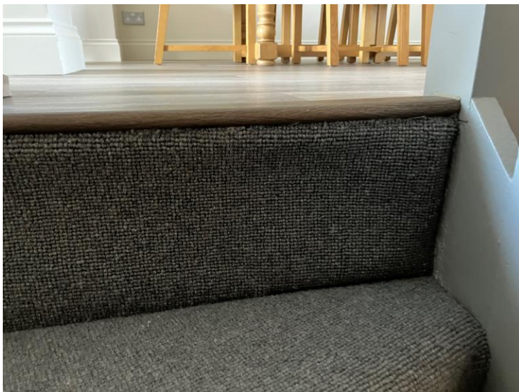
Bulge in carpet where carpet is sitting over original landing nosing. A more appropriate LVT nosing which overhangs the original landing step means that this junction is hidden rather than what is currently installed which left installer no option but to cover the original landing nosing with the carpet. The current carpet can be tidied up in small areas to improve, but the above bulge at the top is unavoidable.
