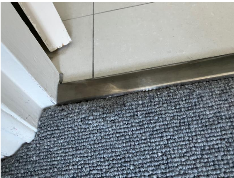
Bulge at en-suite as door bar needs a further securing nail and carpet re-installing.
