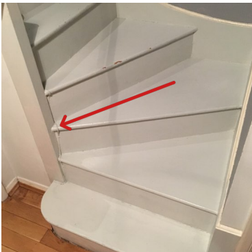
Wire At Side Of Stairs
