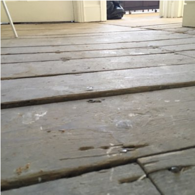
Hallway Uneven Floorboards
