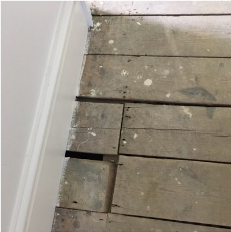
Hallway Uneven / Loose Floorboards
