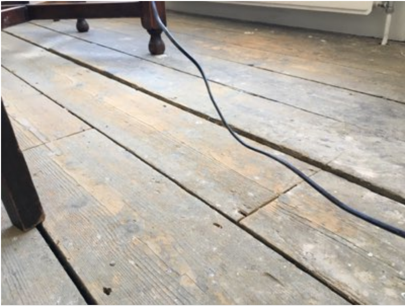
Sitting Room Uneven Floorboards
