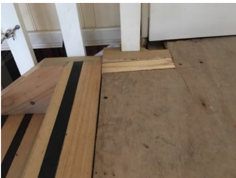
Landing (not being done)
