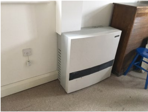
Heater (2 of these are in the Boardroom)
