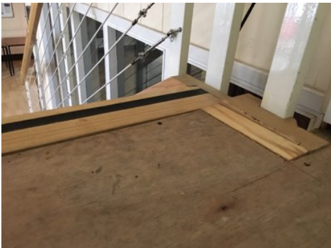
Landing (not being done)
