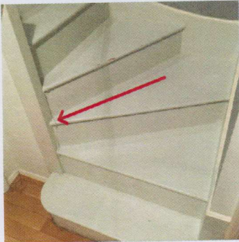
Wire At Side Of Stairs
