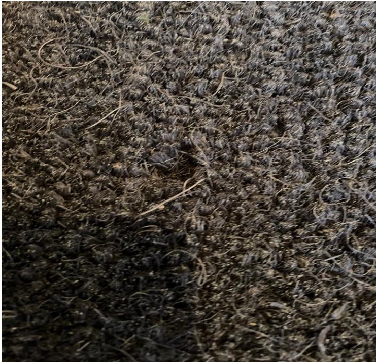
Tufting issue in coir matting – requires replacement
